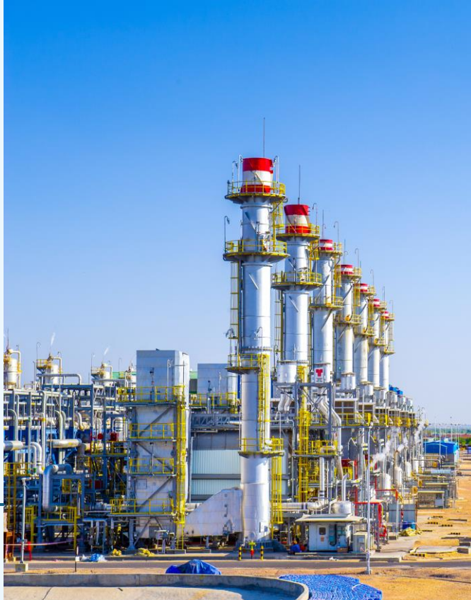
Rajasthan: Mangala Processing Terminal
