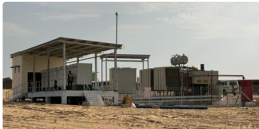
Inverter Control Room
