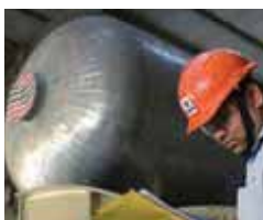
Engineer at Turbine Generator of 2,400 MW power plant, Jharsuguda
