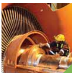
Turbine Generator, Talwandi Sabo project
