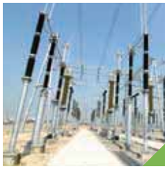
Switchyard, Talwandi Sabo project
