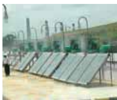
Solar Panels installed at SEL
