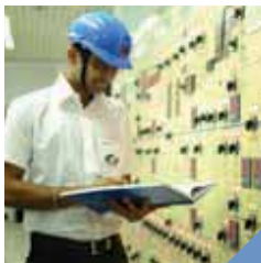
Engineer verifying operating parameters at electrical control room of switchyard, BALCO
