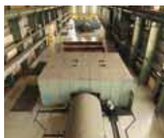
2 units of Turbine and Generator at Chanderiya CPP, HZL
