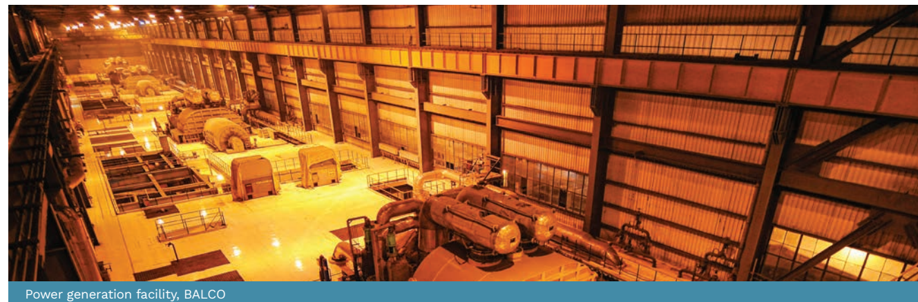
Power generation facility, BALCO
