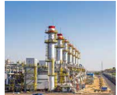
Right: Rajasthan: Steam Turbine Generators at Mangala Processing Terminal
