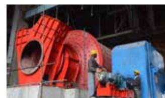
Turbines at Talwandi Sabo power plant
