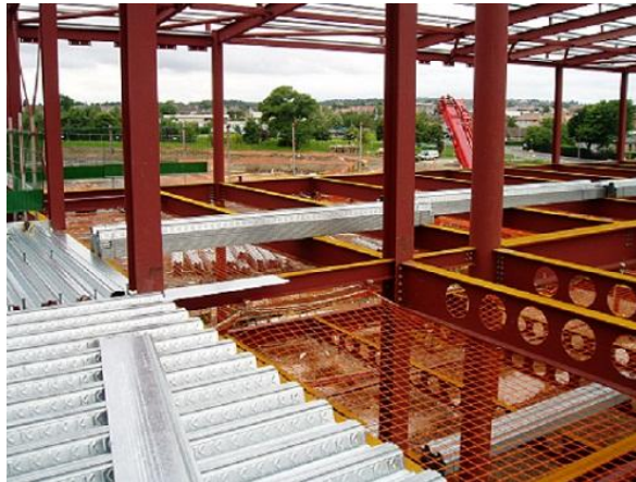
Example of safety nets applied at the “leading edge” on a construction project.
